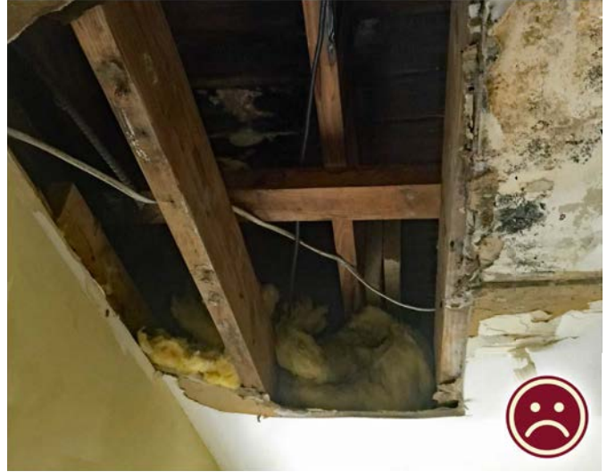
Water damage before the renovation.
