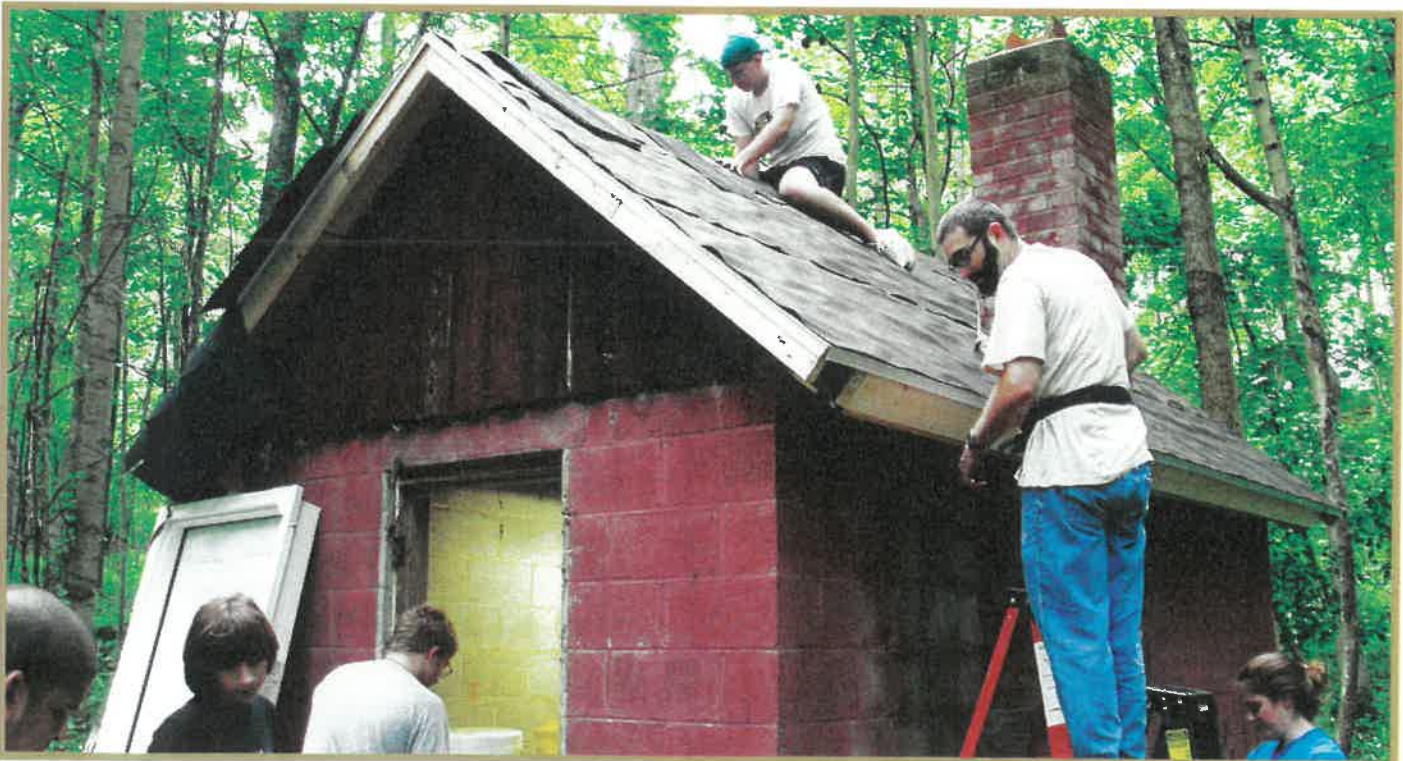
A church youth group renovated the pump house, which was in disrepair for five years.
