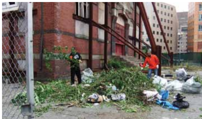
Mission men clean up the area surrounding the Gales School, improving the neighborhood before the Mission even begins construction.
