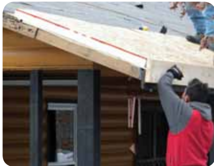
Camp Bennett celebrated its $300,000 renovation this year with an Open House. Thanks to a generous matching grant from the state of Maryland, we were able to renovate and winterize our girls' cabin and lodge and, as seen here, put new roofs on all our 1930s-era buildings.
